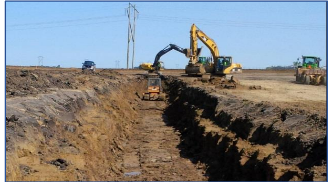
Figure 5. Construction of an engineered seepage cut-off trench on a water storage reservoir (PBS Water Engineering Ltd.).
