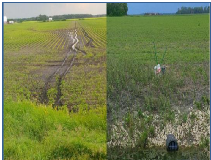
Figure 5. Rutting in wet soils (left) and improved trafficability under drained conditions (right).
