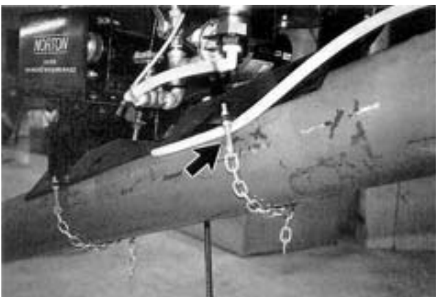
FIGURE 8. Restricted liquid line when Fastened Behind Clamps.
