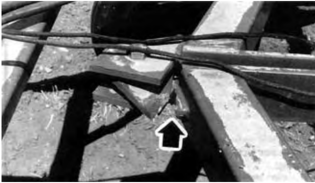
FIGURE 26. Front Pivot Joint Failure.
