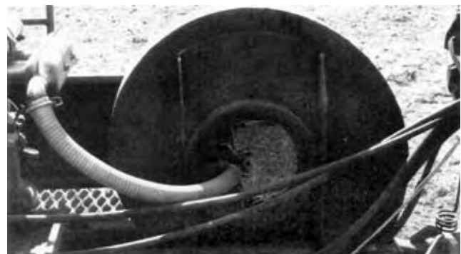
FIGURE 22. Fan Inlet Plugged with Trash.
