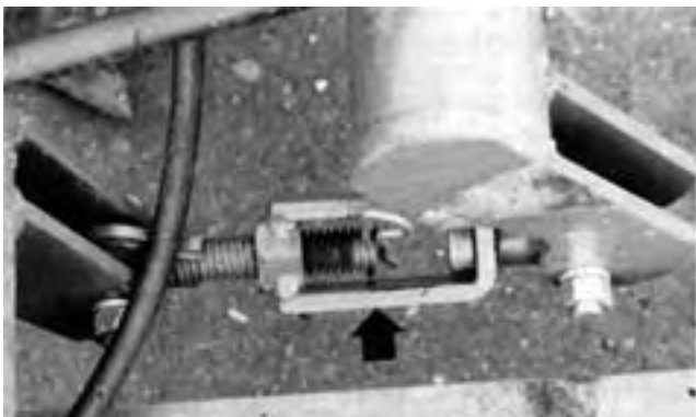
FIGURE 18. Awkward Location of Wing Adjustment Turnbuckles.
