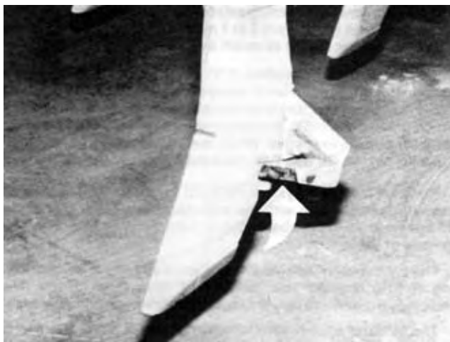
FIGURE 10. Broken Sealer Plate.
