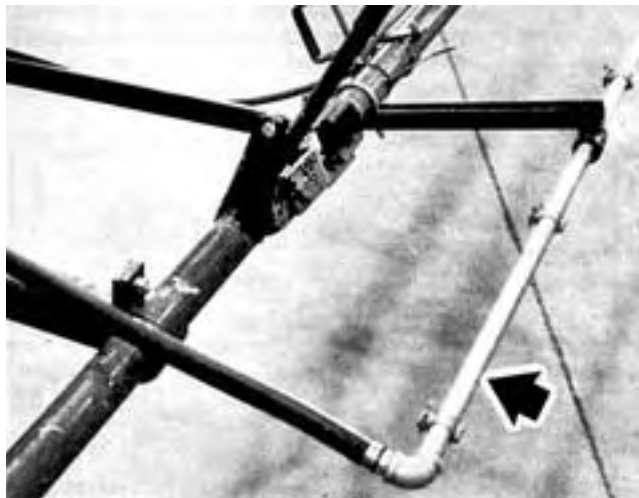
FIGURE 11. Unsupported Section at Centre of 64 mm (2.5 in) Boom Support Rail Assembly.
