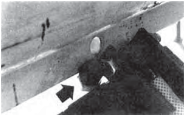
FIGURE 16. Damaged Nozzle Assembly.
