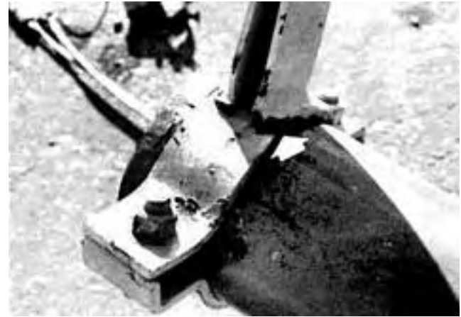
Figure 18. Typical Boom Upright Failure.
