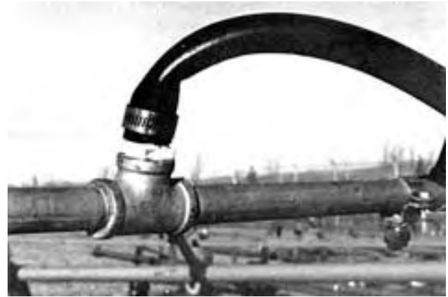
Figure 12. Buckling of Supply Hose at Boom Inlet.
