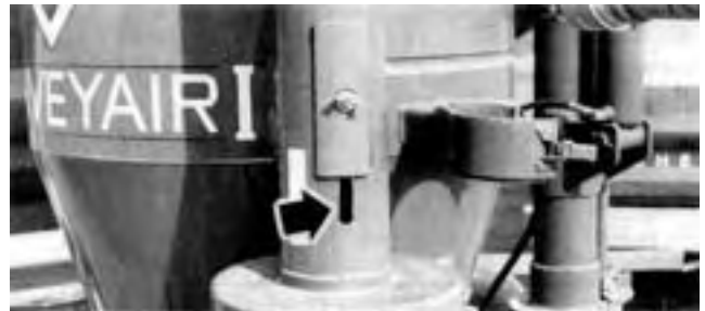
FIGURE 8. Secondary Air Opening Located Above Filter.
