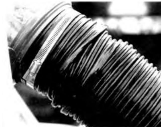
FIGURE 19. Collapsed Vinyl Flex Hose.
