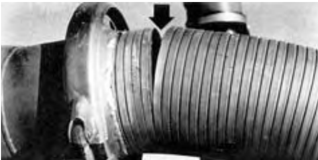
FIGURE 18. Cracked Flexible Piping at Separator Cyclone Inlet.
