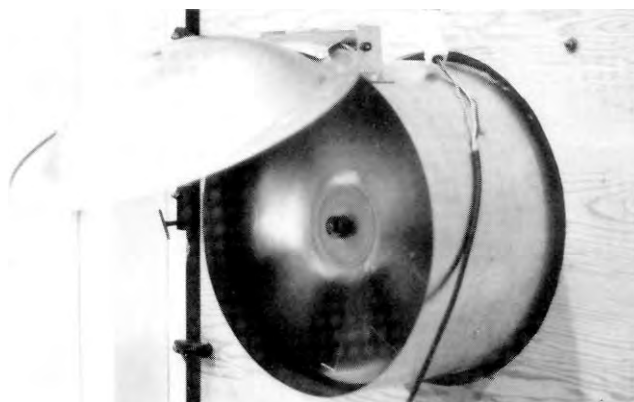
FIGURE 4. Shutter Located on Fan Discharge.
