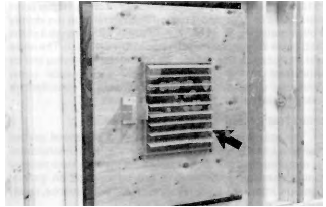
FIGURE 4. Louvres Located on Fan Discharge.
