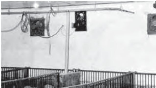
FIGURE 2. The Del-Air A350 Installed.
