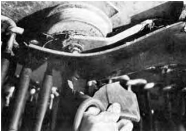
FIGURE 9. Torn Elevator Flighting.
