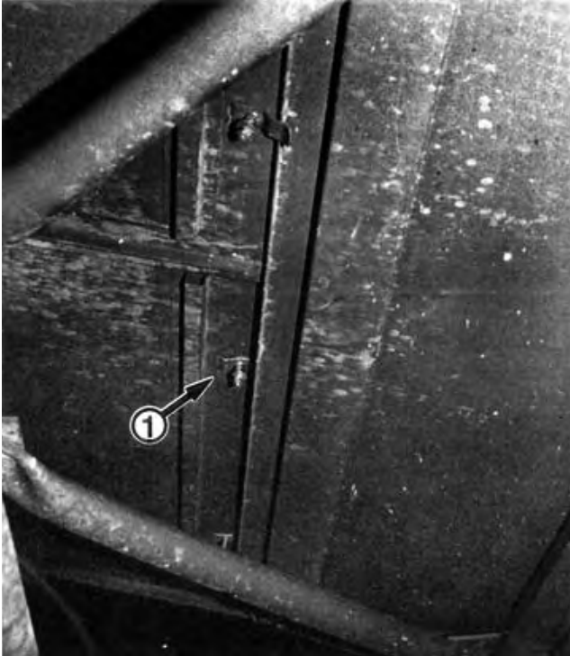
FIGURE 19. Incorrectly Installed Panel (1).
