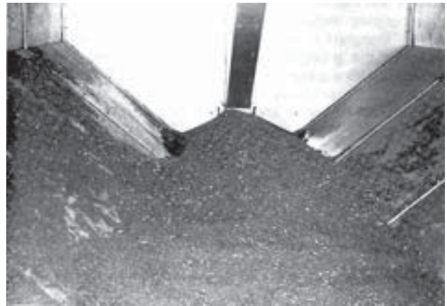
FIGURE 10. Accumulation of Fines in the Cool Air Plenum.
