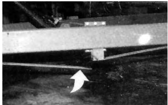
FIGURE 6. Broken Hitch Truss.
