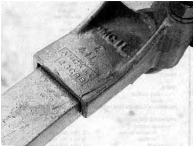
FIGURE 12. Shank Holder Crack.
