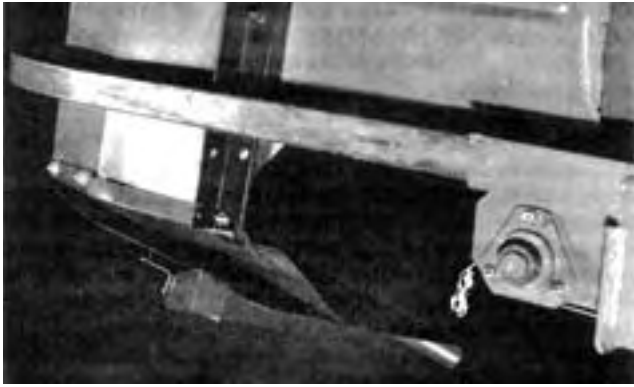
FIGURE 3. Failed Steel Angle.
