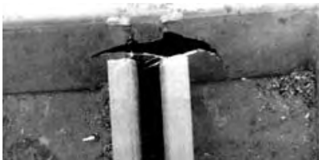
FIGURE 4. Broken Header Tilt Bracket.
