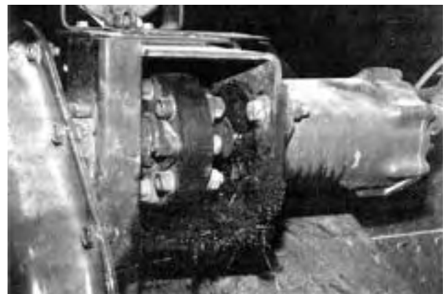
FIGURE 5. Leaking Oil Seal
