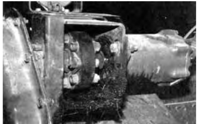
FIGURE 5. Leaking Oil Seal on Hydraulic Motor.
