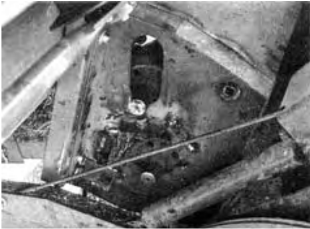
FIGURE 8. Failed Bearing Support Plate.
