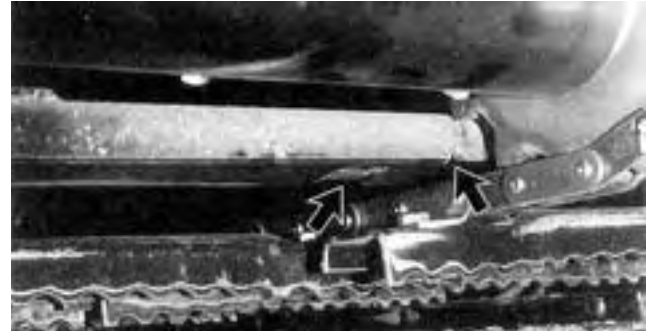
FIGURE 12. Wear on Structural Member Caused from Feeder Chain.
