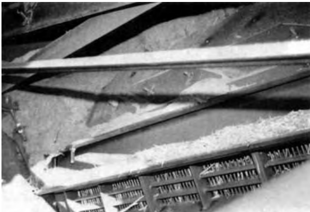
FIGURE 18. Chaff Accumulation Above Rotor Cage.
