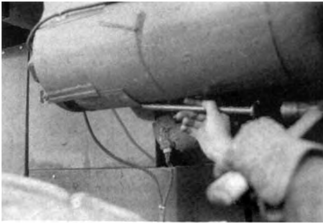
FIGURE 17. Sliding Sump Door.
