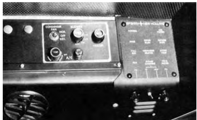
FIGURE 5. Shaft Speed Monitors.
