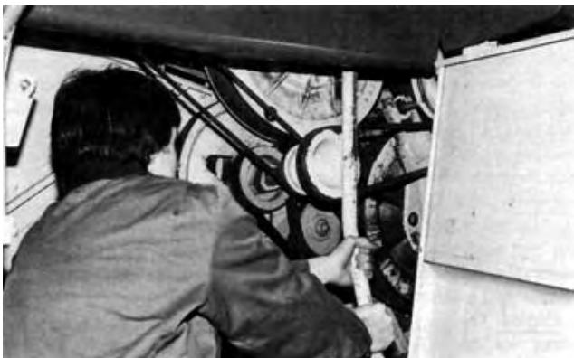
FIGURE 9. Limited Access to the Rotor Drive Rocking Hub.
