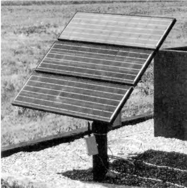
FIGURE 1. Cap 3 Solar Panel
